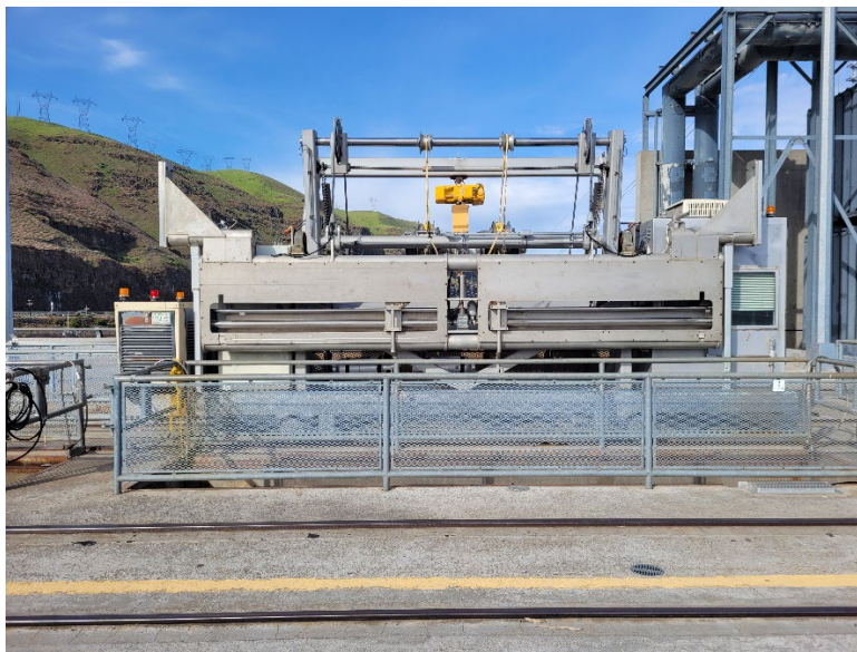
Figure 1: STS camera train
